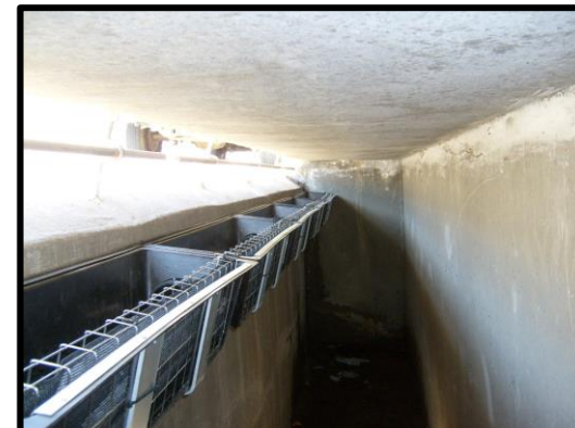
TRC14 - FOG (14' Curb Inlet Filter – Installed)
