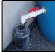
Common Exit Pipe hook-up
