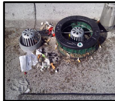
Trash buildup around filter
