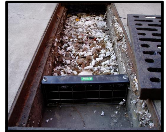
TDAM - FOG Installed in a trench drain
