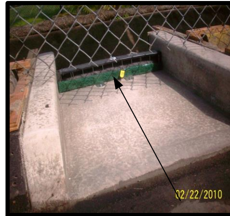
TDAM - BFTG - FOG Installed in a curb
